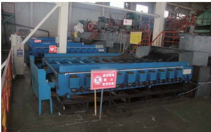
Equipment for recycling fine-graded carbon in Inner Mongolia Pacific Mining Co Ltd.
