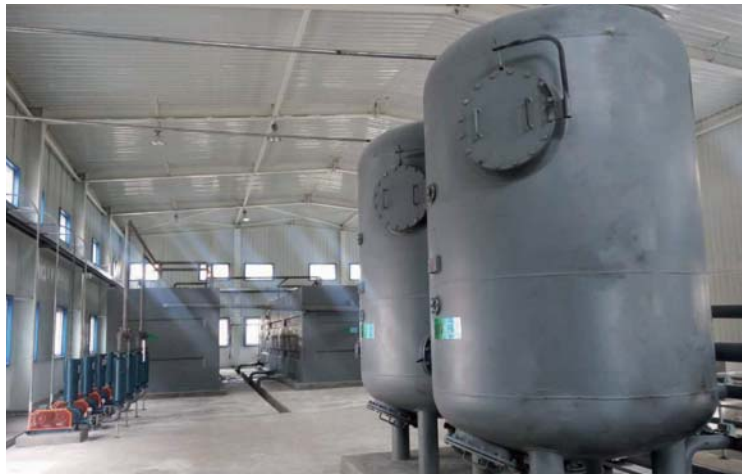
Equipment in newly built wastewater treatment plant of Tibet Huatailong
