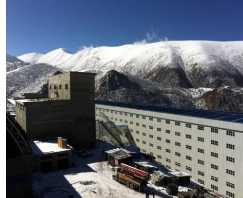
❖ future crushing plant
