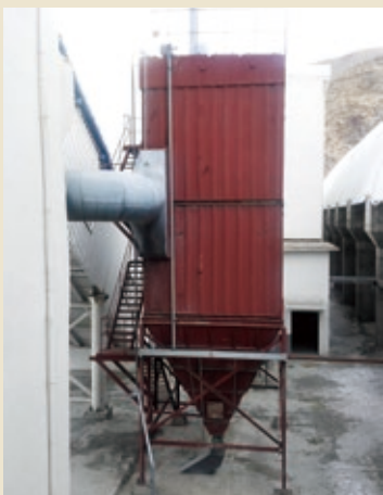
De-dusting system of Phase II plant in Tibet Huatailong
