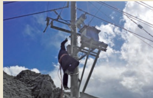
Screener of Tibet Huatailong Inspects Power Lines Earnestly to Make Sure the Smooth Running of Front-line Production
