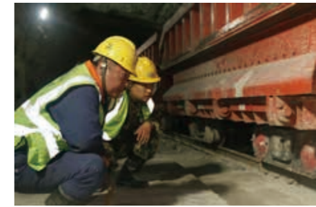
Electromechanical Workers of Jiama underground mine branch was checking the track transport
