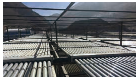
Jiama solar heating system
