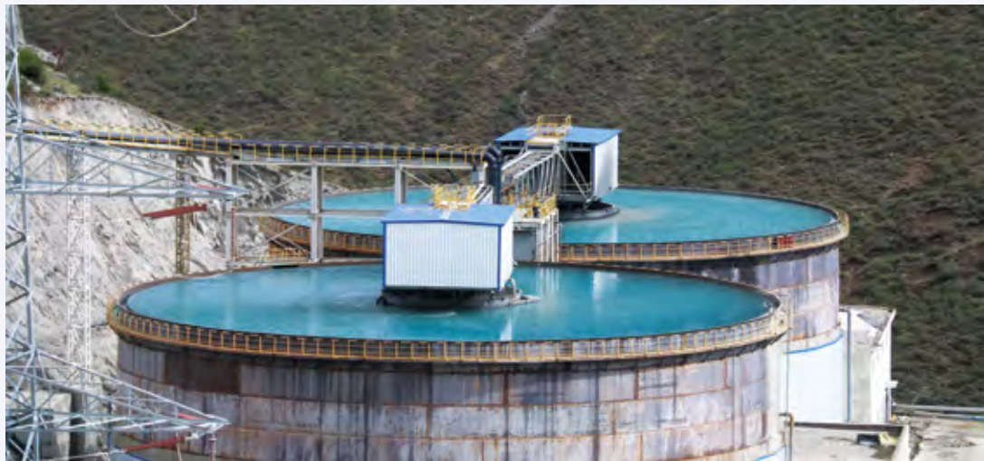
Jiama Mine's newly-built equipment
