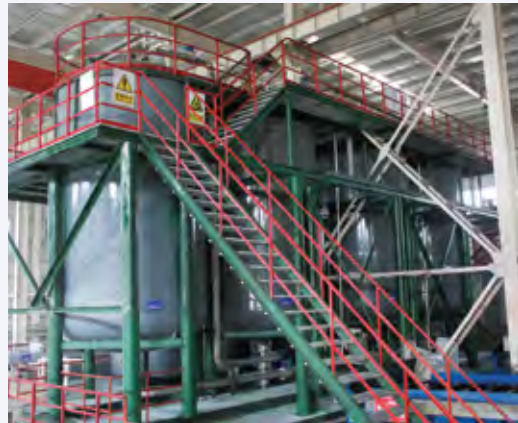
Recovery equipment of heavy metal in Inner Mongolia
