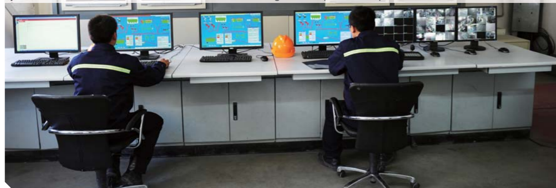
Central control room of Inner Mongolia Pacific
