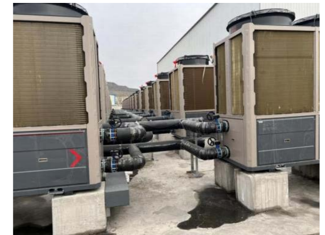
CSH Mine installed air-source heat pumps.
